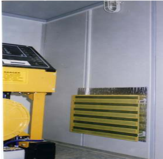
Figure 1: Heating radiant system for industrial applications
