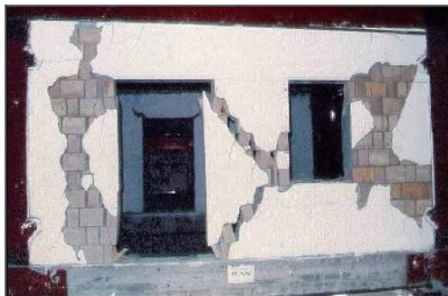
Figure 14 - Damage patterns for ordinary masonry
