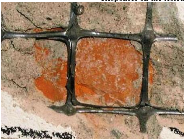
Figure 18 - Failure pattern in Tensar SS20 after 18 dB = 1.96 g
