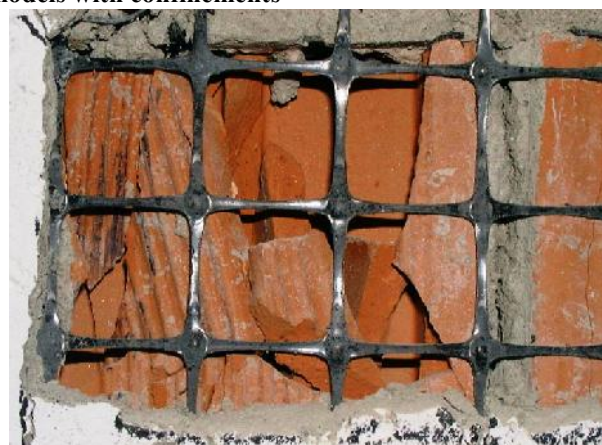
Figure 19 - Failure pattern in Tensar SS20 after 18 dB = 1.96 g
