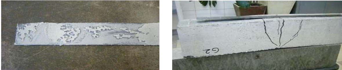
Fig.14 –Detach between plates and concrete.
