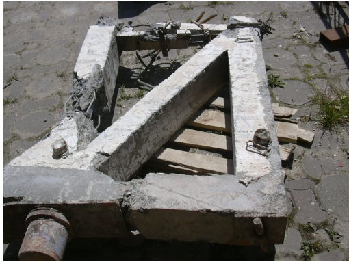
Fig. 8. Reinforcement blockage for prestressing
