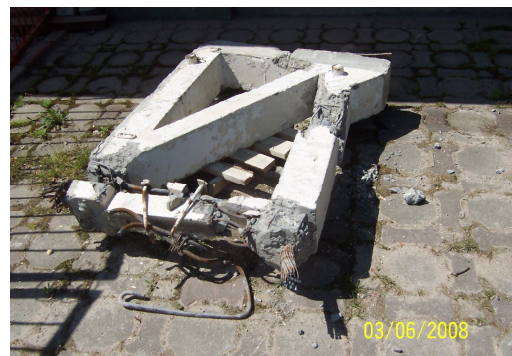
Fig. 7. Stranded wire from soles truss
