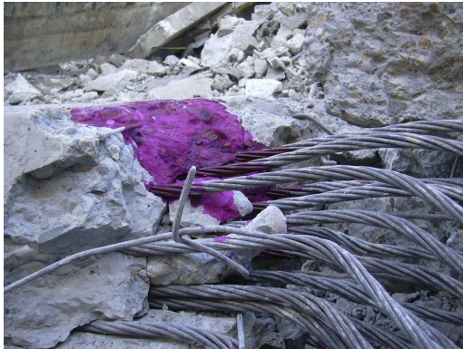
Fig. 10. Alkaline concrete in all beam section
