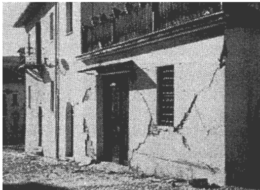
Fig. 3. Degradations of a brickwork construction from Umba-Marc, Italy, during the earthquake of 1997
