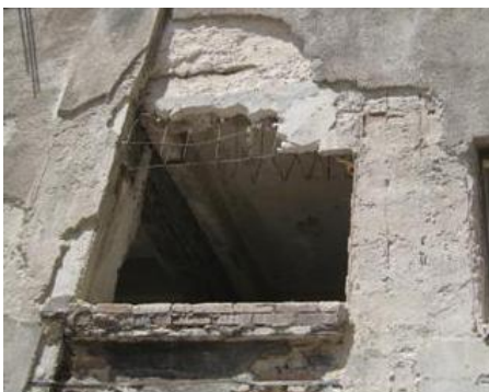
Fig.5. A deteriorated wall
