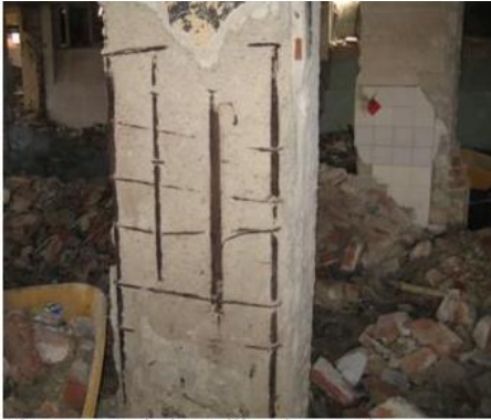
Fig.4. An existing pillar damaged
