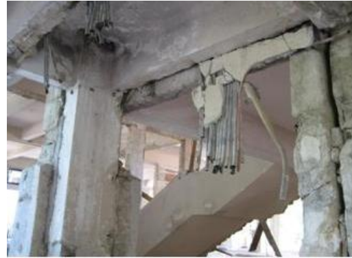
Fig.6. A deteriorated frame of reinforced concrete
