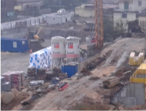
Fig. 3. Image from the execution after heavy rain
