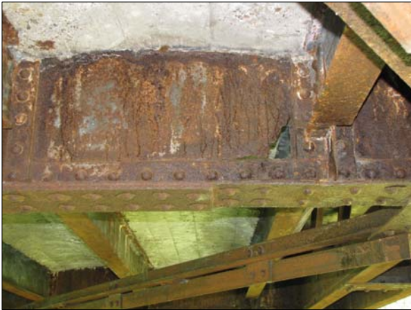
Fig. 8 Corroded cross girder
