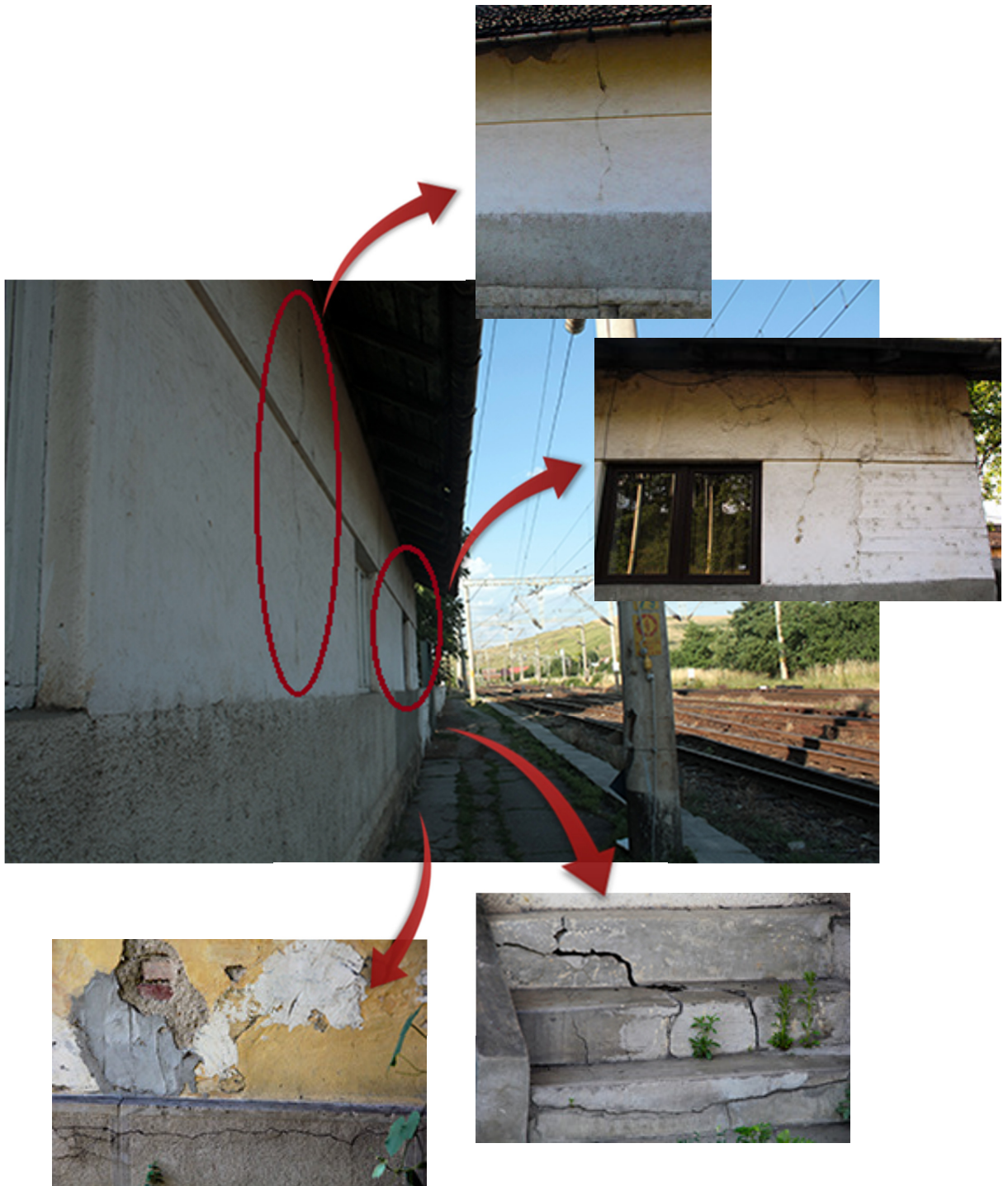
Fig. 5. Dwelling building – damage due to railway traffic
