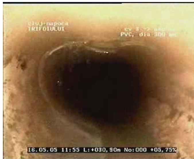
Fig. 7. Severe deformation of the pipe cross section – the sealing is compromised
