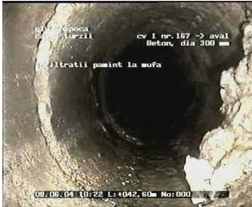
Fig. 2. Faulty joint in a concrete sewer section allowing soil to enter inside the pipe (in the right side of the image)
