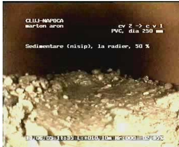
Fig. 6. Deposits of sediments – 50% of the pipe cross sections is unusable due to sediments
