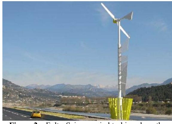
Figure 2 – Eoltec Scirocco wind turbine along the highway in France
