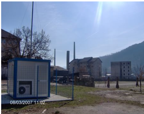
Fig. 2. Industrial type of monitoring station
