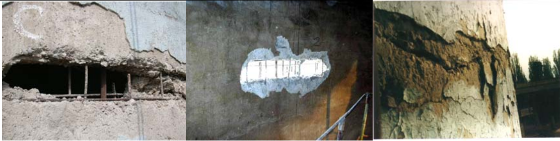
Fig.19 Hole, view from outside Fig.20 Hole, view from inside Fig.21 Deep damages in concrete
