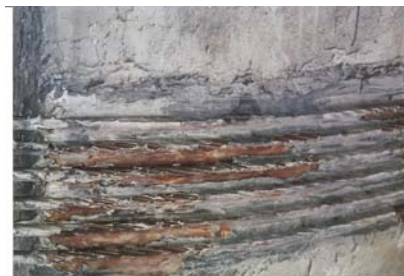
Fig.5 Strands on the bearing zone
