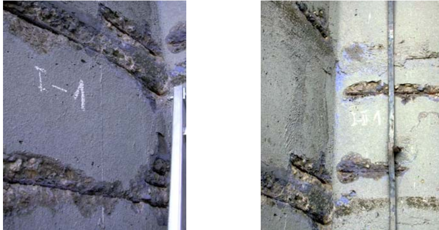
Fig. 24, 25 Expelled concrete in zone with reduced concrete cover
