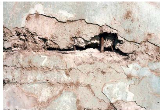
Fig.18 Detached bars cover, cavities
