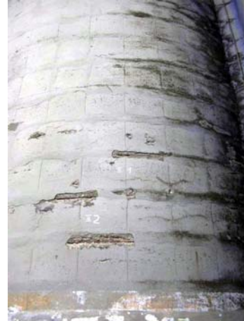
Fig.16 Deteriorations on external cell surface
