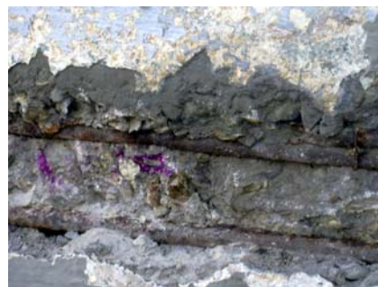
Fig.23 In-deep reinforcement corrosion
