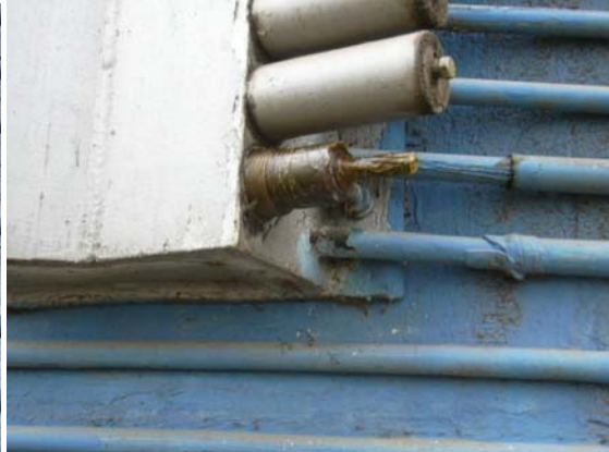
Fig.12 Grease state of anchorage after removing sleeve nut
