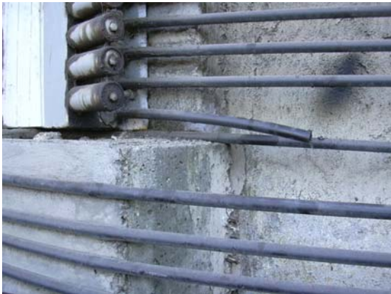
Fig. 11 Actual view of strands in tube and anchorage sleeve nuts
