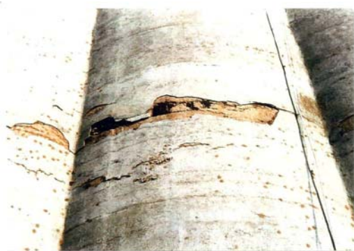
Fig.17 Deep deteriorations in concrete
