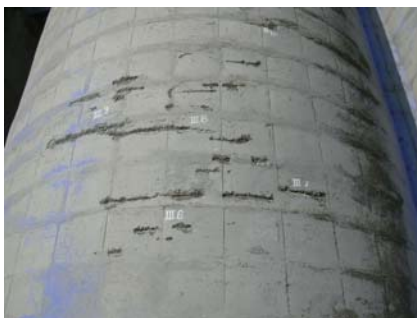
Fig.22 View of outside affected zones
