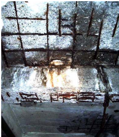
Fig. 7. Floor with corroded reinforcement
