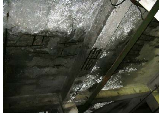
Fig. 1. Damaged floor due to the presence of water vapour
