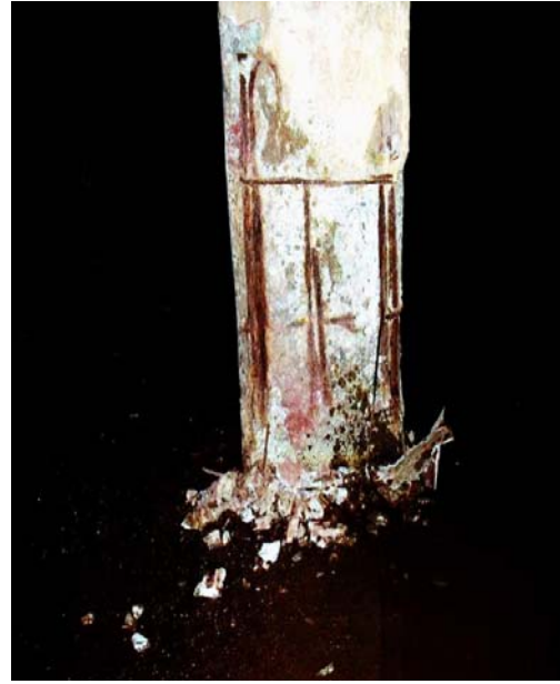
Fig. 5. The column base strongly corroded due to permanent water from the basement
