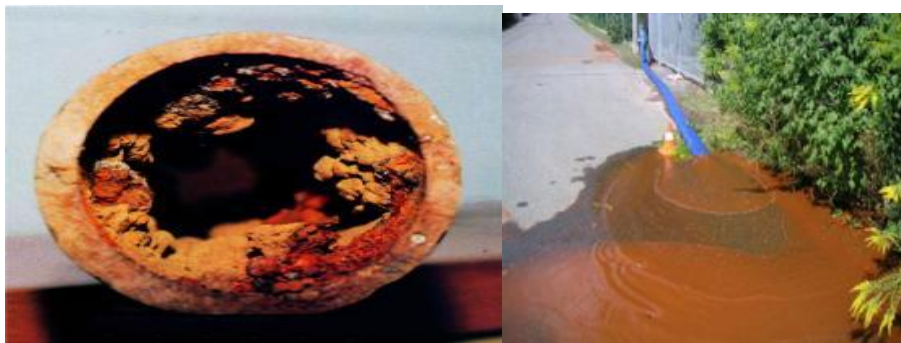
Figure 1: Examples of rust the pipes
