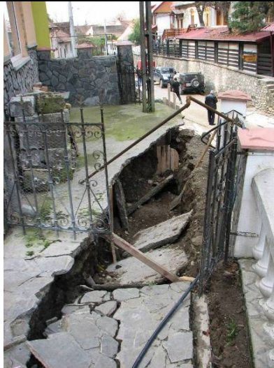
Fig. 5 Crashing of portions of land behind the retaining wall
