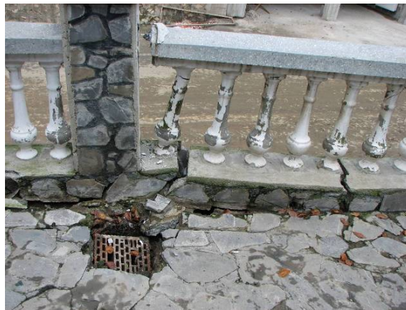
Fig. 4 Cracks in the protection bulwark area
