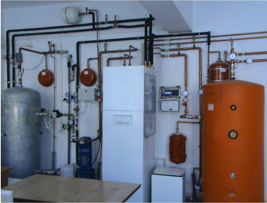
Fig. 4 The heat pump between the cold and the warm water tank
