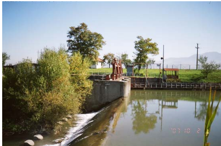
Fig. 3. Weir and gates Turcu
