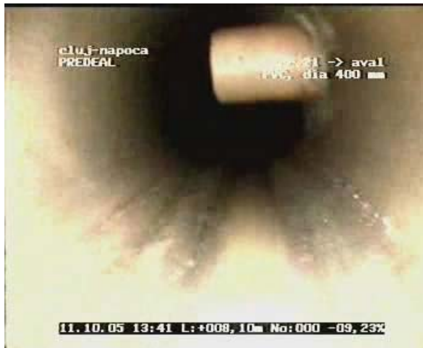
Fig. 4. Protruding lateral inside sewer main prevents the camera robot to advance along the pipe [2]
