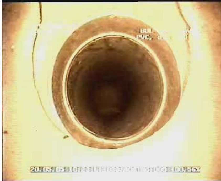
Fig. 1. Cracks in the wall of a PVC sewer main at a lateral joint due to uneven soil compaction and the lateral acting as a lever
